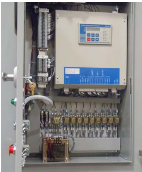
HRVS-DN Digital Control Module located in isolated low voltage compartment
