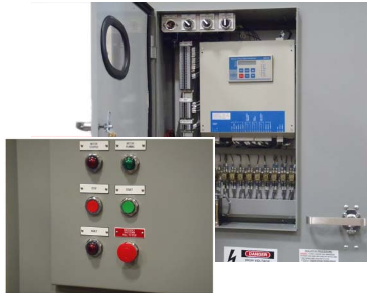
Door Mounted Pilot Devices
