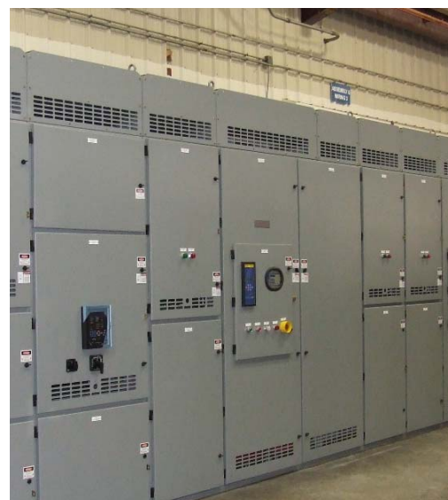
Metal-clad type construction
