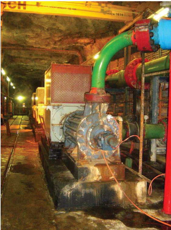
4 x 6.6KV / 1.5MW at 2100 and 1200 meters underground
