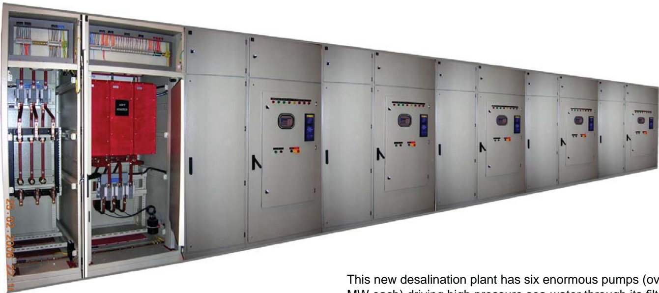
HRVS-DN 6600V / 400 A for 6 desalination pumps
